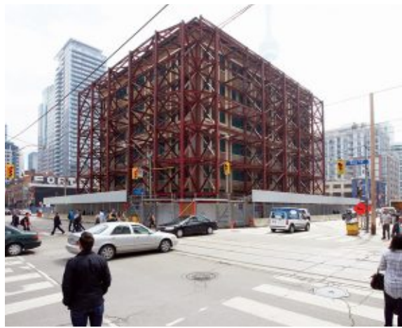
LENSCAPE INCORPORATED—The steel truss support system was designed by Jablonsky AST and Partners.
